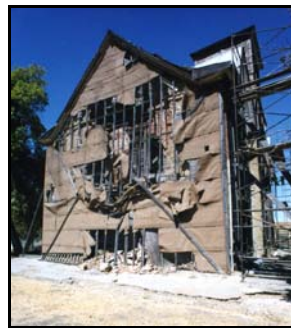
The south wall is next on the repair list once the foundations are secure.
