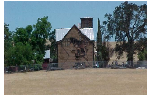
The south wall remains unrepaired today. Rain is a constant threat to the house.
