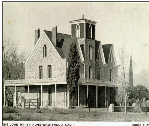
South wall of the Stone House before its collapse in the 1970s. Photo c 1930s. Courtesy of Carol Jensen
