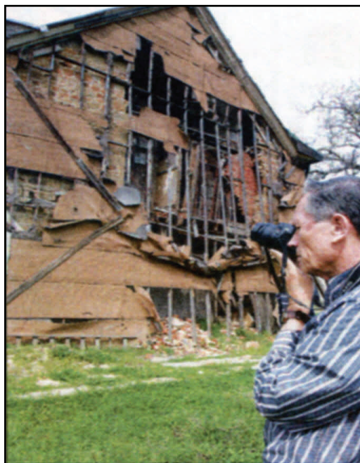
Bill Mero, JMHT Board member and newsletter editor, records the deterioration of the south wall of the historic Marsh House. Photo by J. Chapman/staff, courtesy of Discover the Delta, Bay Area News Group.
